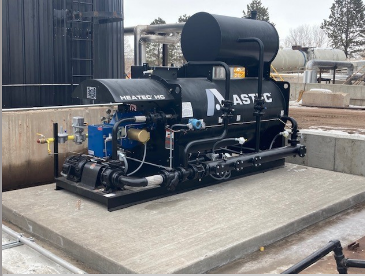
New hot oil heater.
