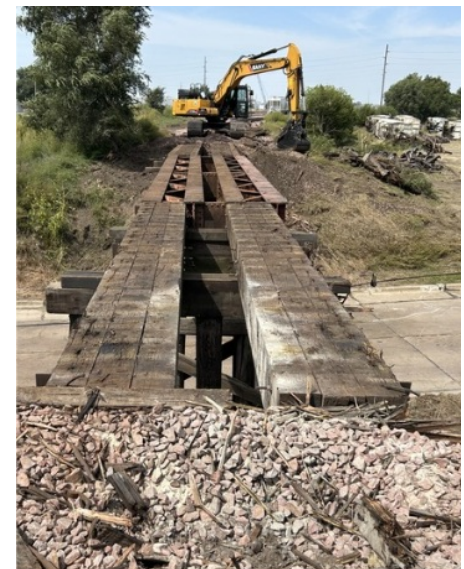
Rail bridge damage- overcoming adversity through creative solutions and teamwork
