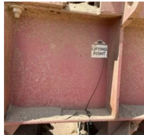
A cracked beam at a plant - one of life's many curve balls
